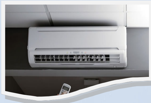
Air-conditioning, Galaxy Arcade, G-11
